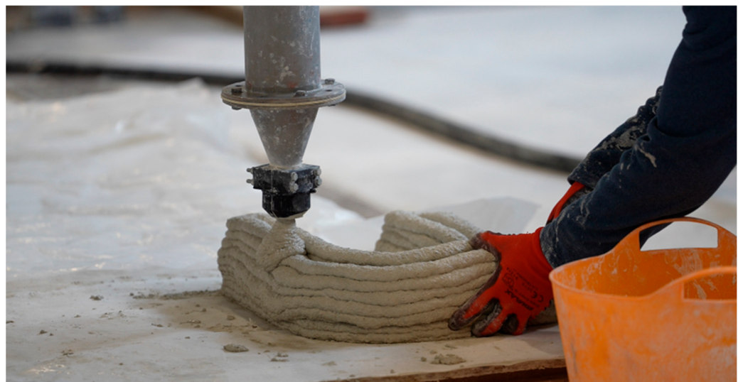
Figure 5. Example of failed extrusion-based 3D concrete printing, illustrating typical instability and buildability issues associated with non-standard or recycled aggregates.
