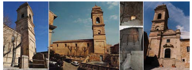
Figure 7. Orbitable 3D model obtained from the processing of aerial photos taken by drone: overall views and detailed views of damage to the roof and façade.
