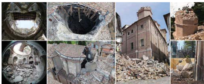
Figure 1. The Church of Santa Maria in Via after the earthquake: collapse of the interior camorcellona dome, roof, and bell tower.
