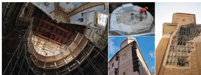
Figure 5. Some pictures of the operations to secure the church: interior drum and dome, corner and top of the bell tower, left side of the façade.
