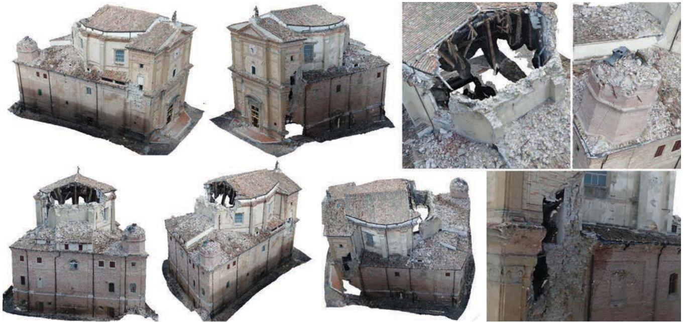
Figure 6. Orbitable 3D model obtained from the processing of aerial photos taken by drone: overall views and detailed views of damage to the roof and façade.
