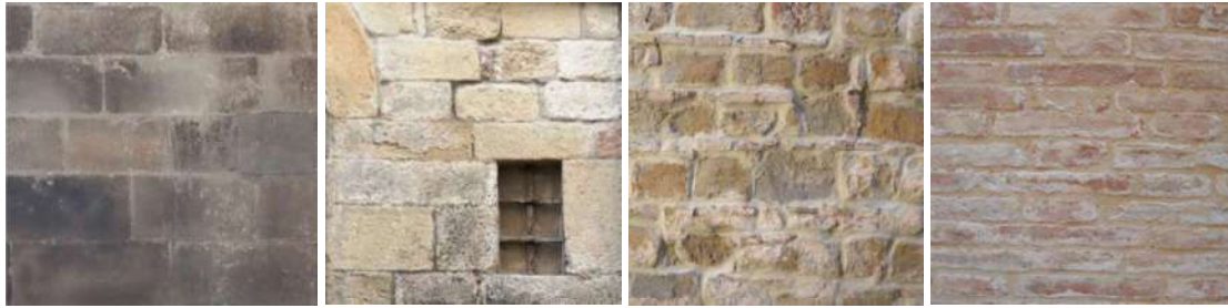
Figure 9: The most common types of masonry in Camerino: 1 - f) Masonry with square stone blocks; 2- e) Regular-block masonry of soft stone (tuff, calcarenite, etc.); 3 - c) Split stone masonry with good texture; 4 - g) Solid brick masonry and lime mortar.
