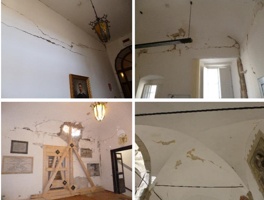
Figure 2: Examples of the damages in “Portico Varano” after the 2016 Central Italy earthquakes.
