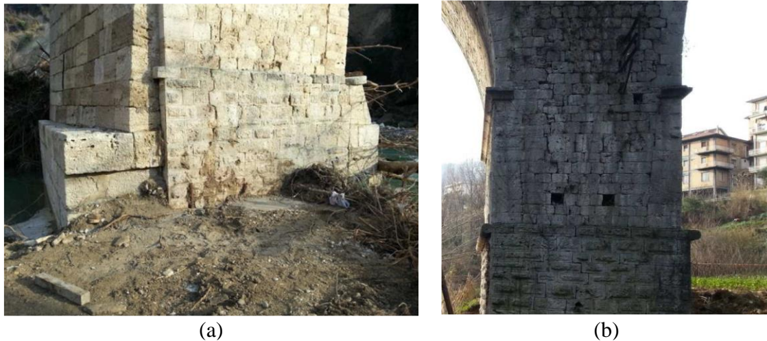
Figure 4. (a) crack pattern at the bottom of pier P1; (b) cracks of pier P3.
