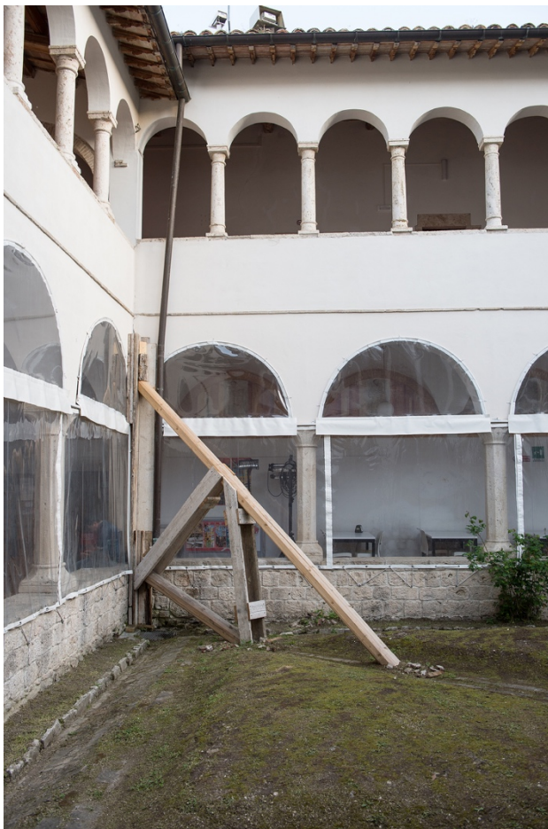
Figure 2. Emergency action for the safety of the main cloister after the earthquakes of August 2016
