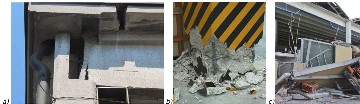
Figure 59: Collapse due to: a) insufficient support length between beam and column, b) collapse in correspondence of the column-to-foundation joint, c) collapse of the cladding panels.
