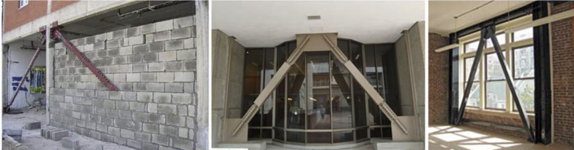
Figure 23: Example of retrofit of r.c. vertical structure with BRB and traditional bracing systems.
