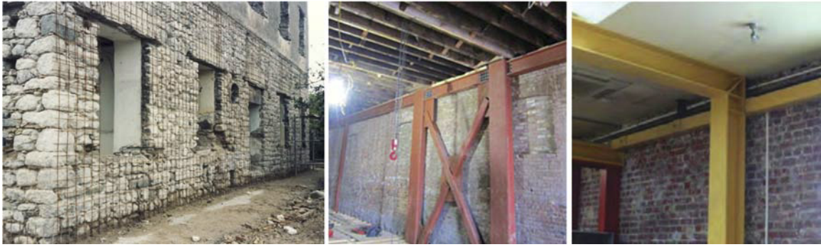
Figure 22: Rehabilitation of masonry walls: with steel mesh and shotcrete, steel braces, MRF steel frame.
