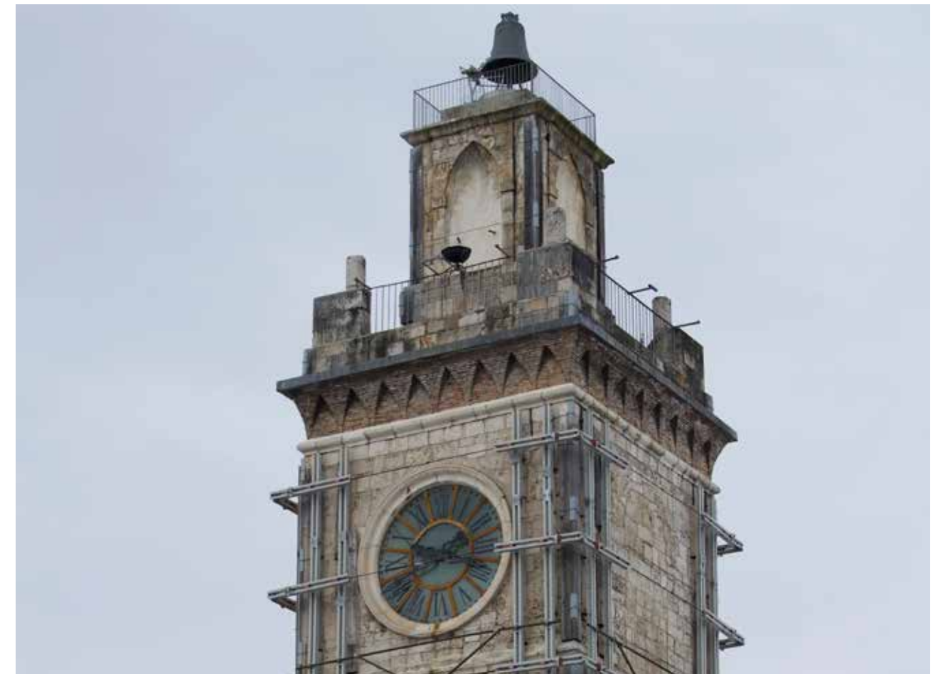
Fig. 1 L'Aquila on April 6, 2009, had an earthquake with a devastating impact on the city's historic center.
