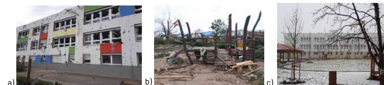
Fig. 6 - Kindergarten: damage after the hit (a), destroyed playground (b), building after reconstruction (c). Source: https://www.mnves.cz/projekty/opravy-budov-po-tornadu-materska-skola/
