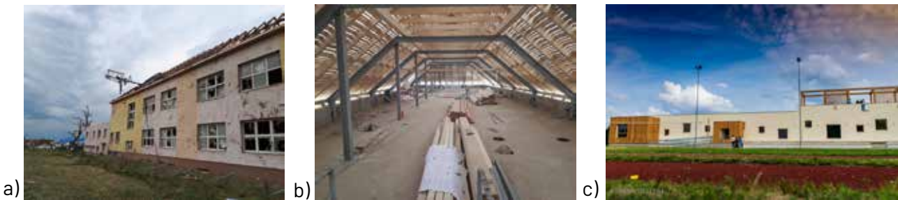
Fig. 10 Doctors' House: damage after the hit (a,b), building after almost completed reconstruction (c). Source: https://www.mnves.cz/projekty/projekt-1/
