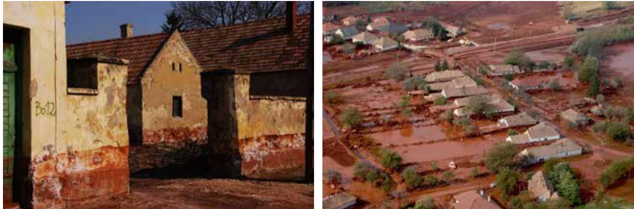
Fig. 3-4 Traces of red mud on the wall of a house in Kolontár and its surroundings (source: Csóka, 2021a)
