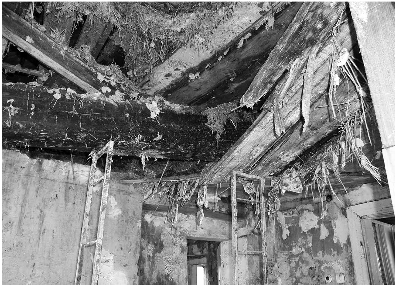
Fig.2 Failed biodegraded timber floor joists in a historic house in Prague Troja during the 2002 flood, (the house was totally immersed in water). © M.Drdáček
