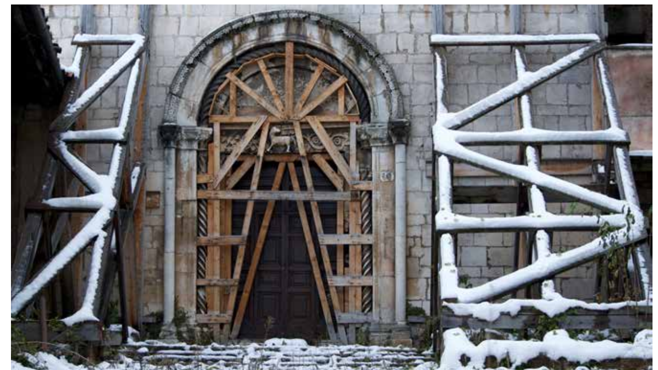
Fig.2 The earthquake produced a severe damage in the city.
