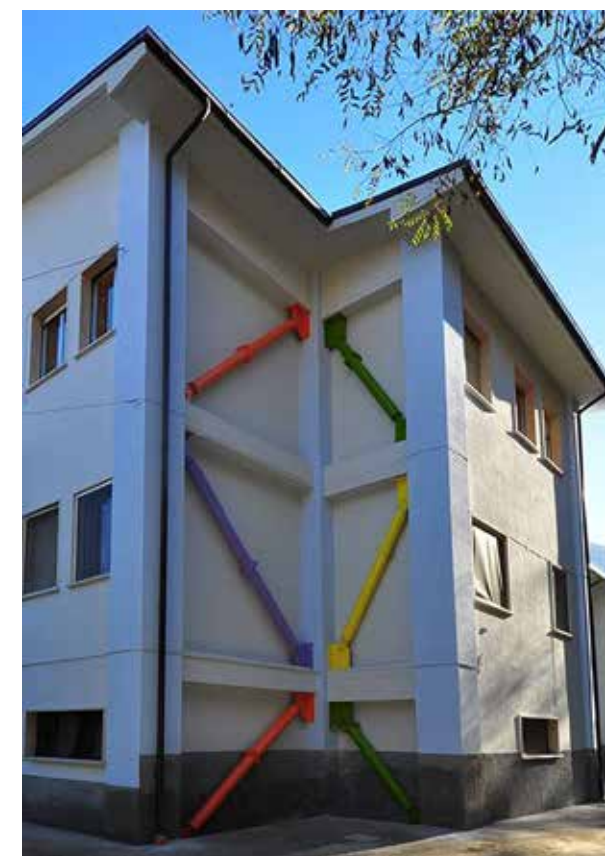
Fig. 3 Example of exposed dissipative braces in an existing structure.
