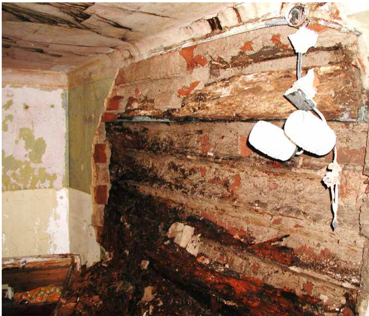
Fig. 2 A timbered wall exposed by the collapse of a brick lining wall. © M. Drdáký
