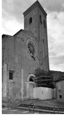
Fig. 1. Façade and bell tower view of the San Zenone Church (Fermo, Italy).
