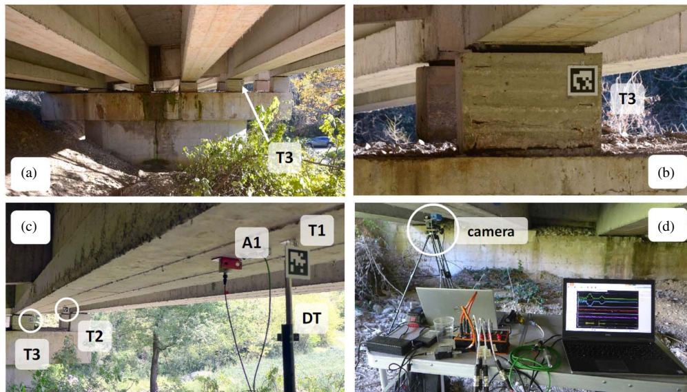
Fig. 6. View of the considered case study: (a) pier as seen under the monitored span with indication of the position of the assumed stationary target T3; (b) detail of the pier cap with Target T3; (c) view of the three targets (T1 at the midspan, T2 at the 3/4 span, and T3 at the pier), DT and accelerometer (A1) at the midspan; and (d) video camera and acquisition system.
