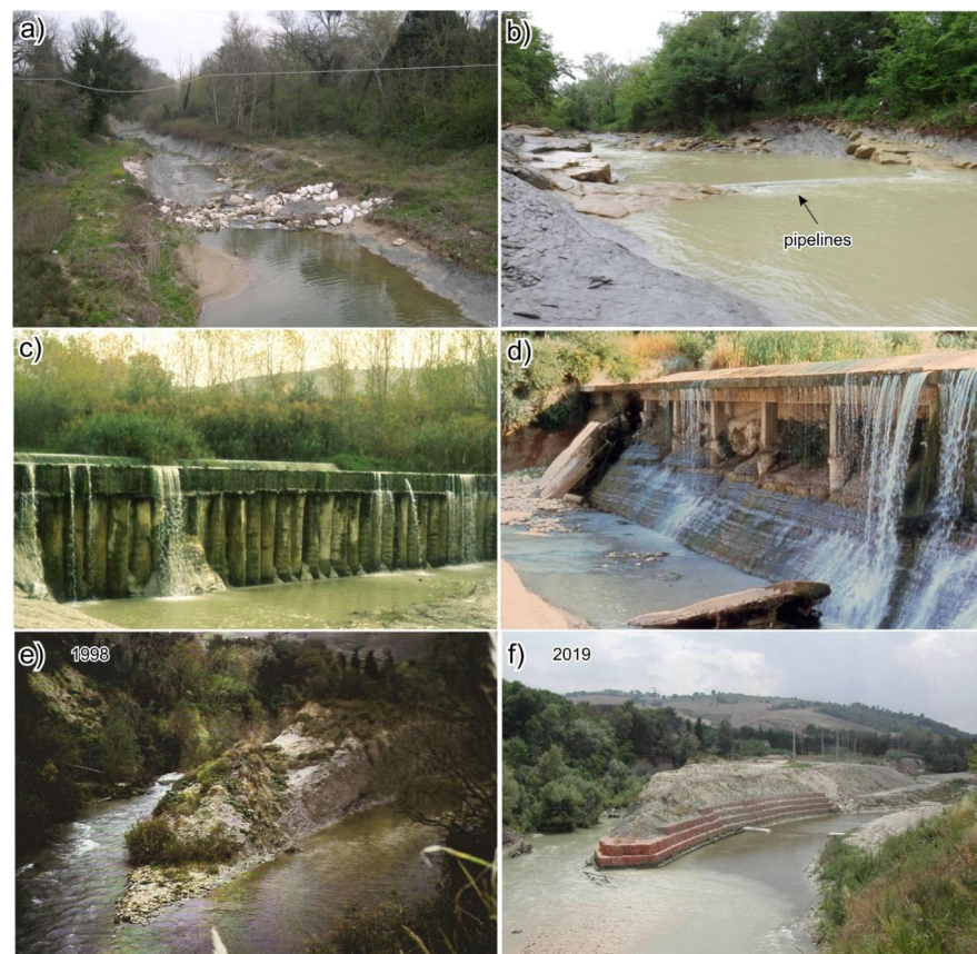
Figure 2. Deepening phenomena observed along some river reaches of the study area: (a,b) recent thalweg erosion along the Chienti River (in the second image, three pipelines have been exposed by erosion); (c,d) deepening phenomena occurred in correspondence of two check dams (Tenna and Potenza River respectively) during the last 20 years; (e,f) river incision occurred in just over 20 years in correspondence of the wastewater treatment plant of Tolentino (C2—Chienti River).
