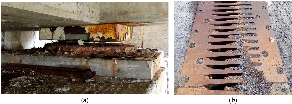
Figure 1. (a) Typical consequences of the expansion joints permeability: degradation and corrosion of a cylindrical hinge bearing device. (b) Debris and materials accumulation within an expansion joint compromising its functionality.
