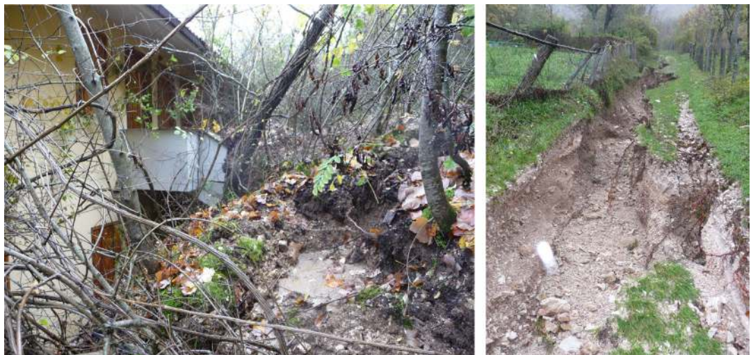
Figure 7 - Effects of the recent debris-flow (left) and siphoning phenomena (right) where the water from the upper parts of the slope seeps into the first subsoil, goes under pressure and rises again pushing, deforming and eroding the soil (images from the Ussita Municipality archive).
