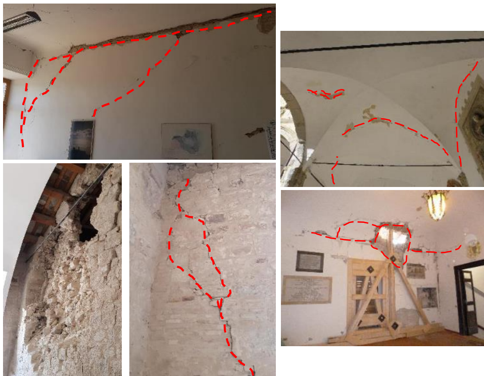
Figure 46 : damages after 2016 central Italy earthquake
