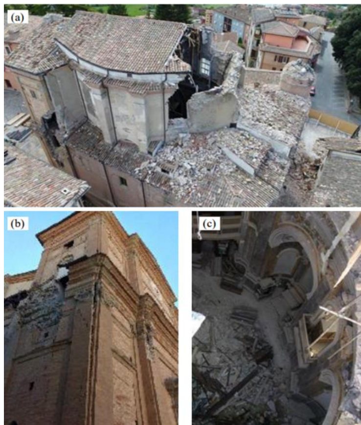
Figure 81 : Damages occurred in the Santa Maria in Via church after the 2016 seismic sequence (a) collapses of the roof of the tiburium and of the bell tower, (b) damages on the lateral part of the façade, and (c) detail of the collapse of the fake dome.
