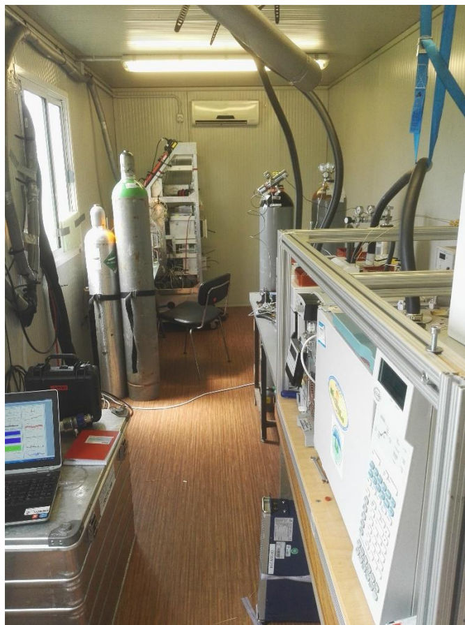
Figure 5.6: Sampling instruments inside the container.
